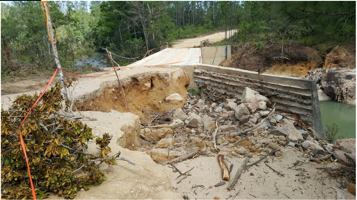
Bridge on the access road to the Las Cuevas plots was washed out by Hurricane Earl in August 2016.
